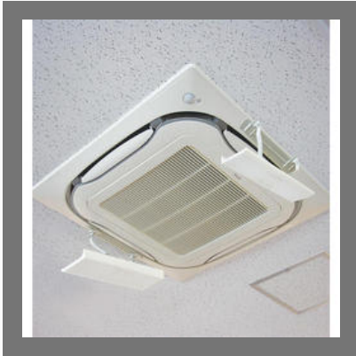
Central Electric Air Conditioner
